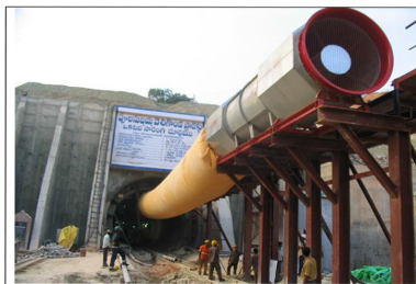
BLOWER PVC DUCTING
